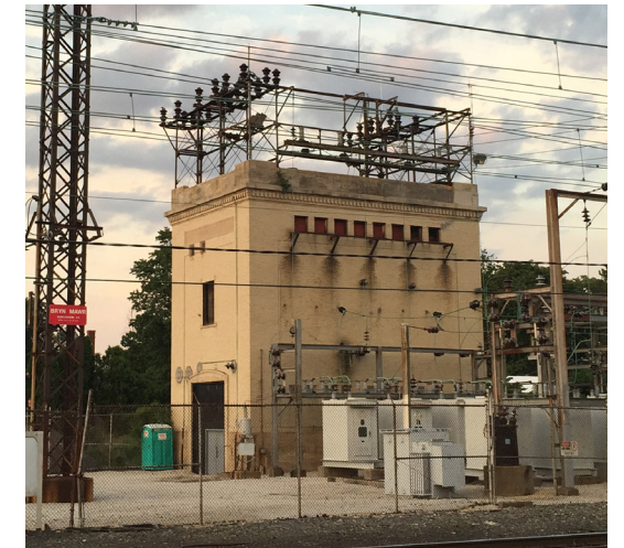
Bryn Mawr Substation
