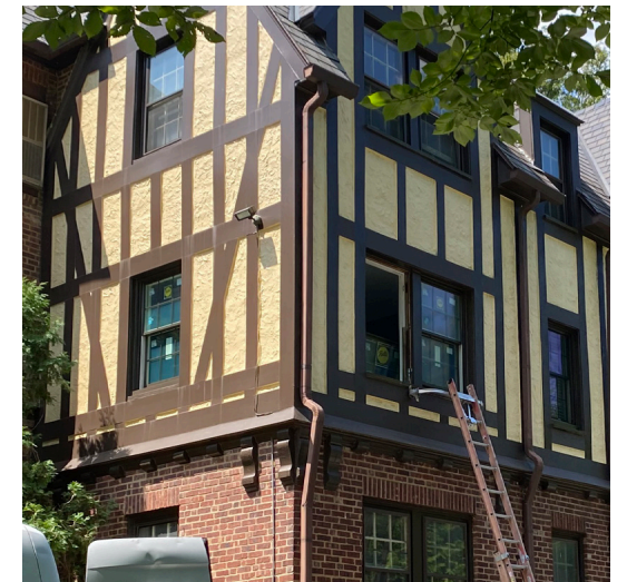
5.19. An inappropriate window replacement at York Lynne Manor.
