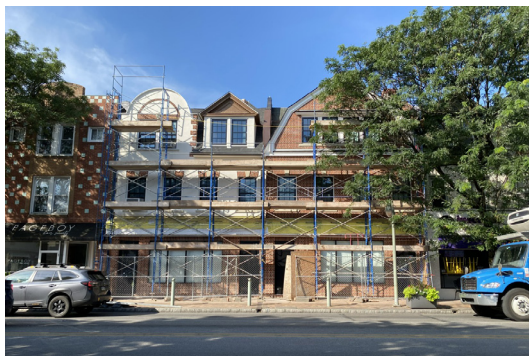
5.8-5.10. The reconstruction of two historic “Colonial Block” facades in downtown Ardmore did not follow the approved plans in terms of proportions, window placement, cornices, and other details. HARB sought to ensure that the work matched the original facade (top) as closely as possible. Work could not be adequately observed while scaffolding was tarped (center), and was only revealed to be out of keeping with the approved plans once tarps were removed (bottom).
